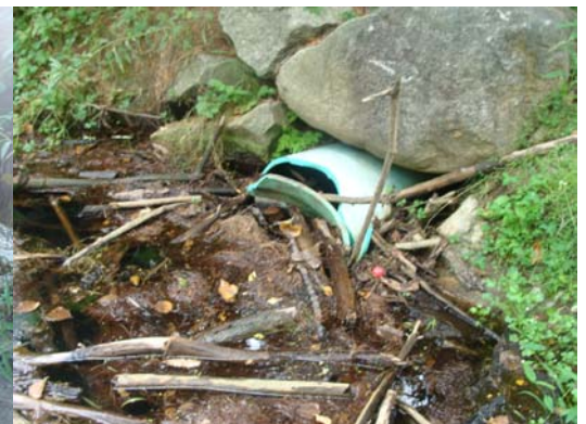
Clogged Culvert-Russell Road
