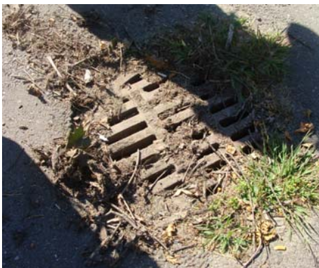
Clogged Storm Drain-Bennett Ave.
