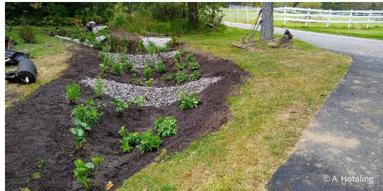
Aerial diagram (top left) with conceptual (top right) and installed (bottom) design of a vegetated swale with check dams for a residential property on Pleasant Lake, NH.
