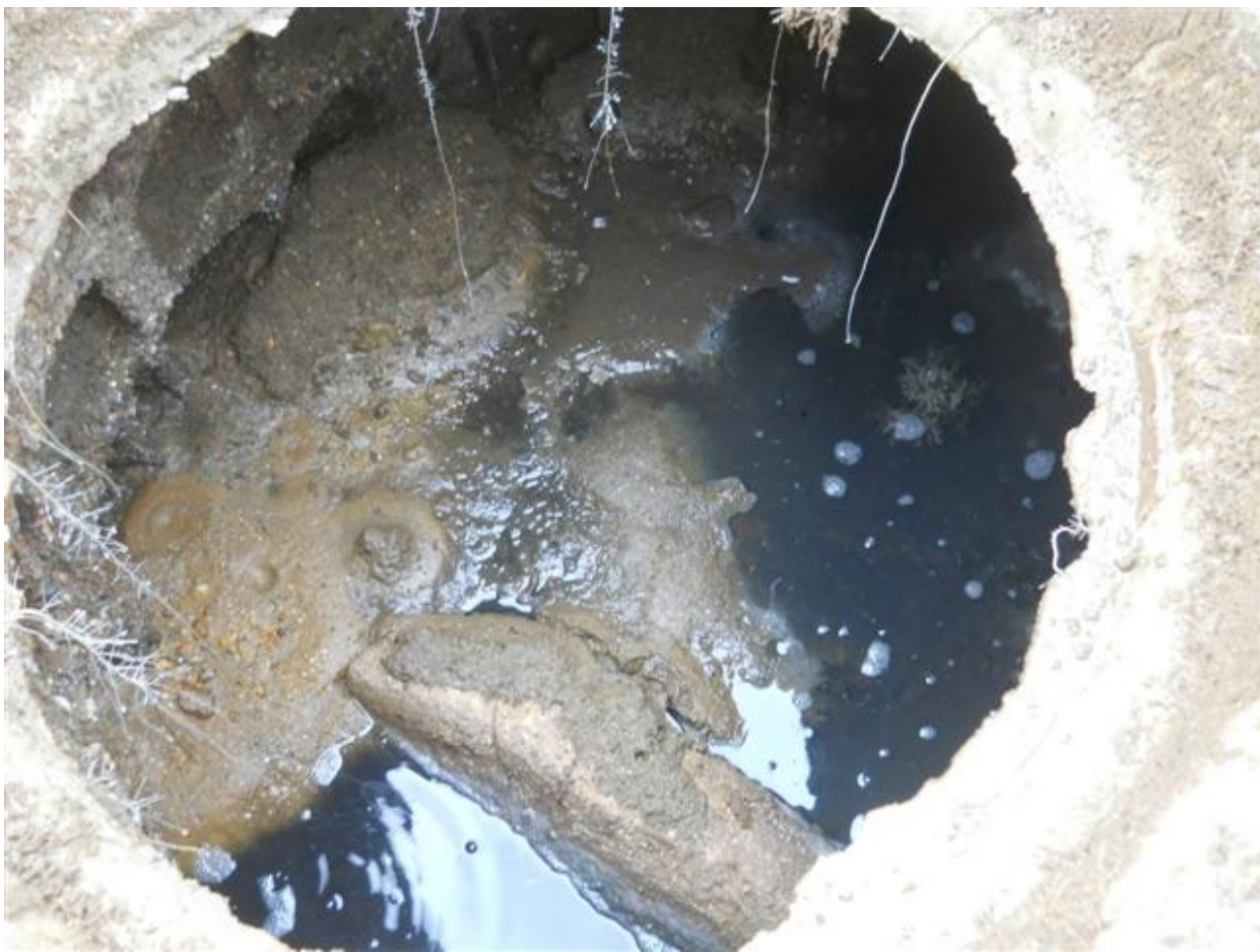
Figure 3. A septic dry well in New Hampshire in poor condition. Photo Credit: Peter C. Russell (Russell Inspection Services) via InterNACHI Inspection Community .
