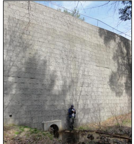
Figure 13: Retaining wall and fill, with small culvert for stream, blocking the floodplain beneath a road crossing. Photo: K. Feindel, Maine DEP.
