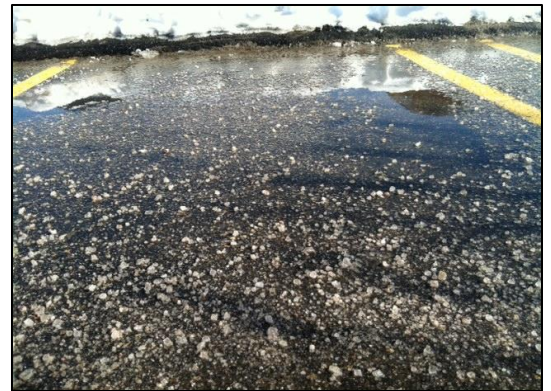
Figure 17: Rock salt applied to a watershed parking lot. Photo, J. Edgerton.
