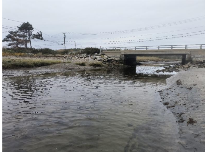
PC-OUT during wet weather on 10/14/2025.
